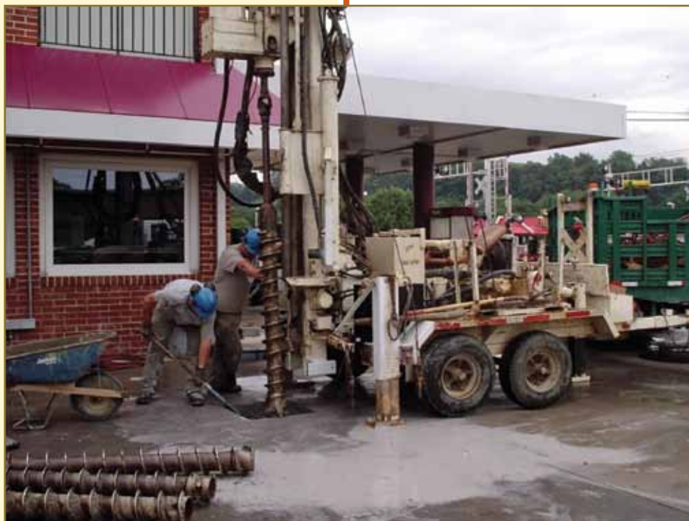
Fig. 3. A drill rig capable of drilling to 100 feet or more with hollow stem augers, rock coring equipment or air rotary equipment for collection of soil, rock, and water samples.
